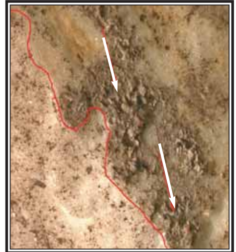
Figure 8: The chiseled spall area (left) fractured through areas of the remnant mortar (white arrows) on the back side, indicating the spall happened after the mortar had hardened.
